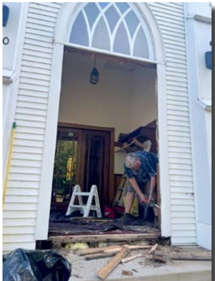
Preparing the opening for our new doors. This work should take about one week.
