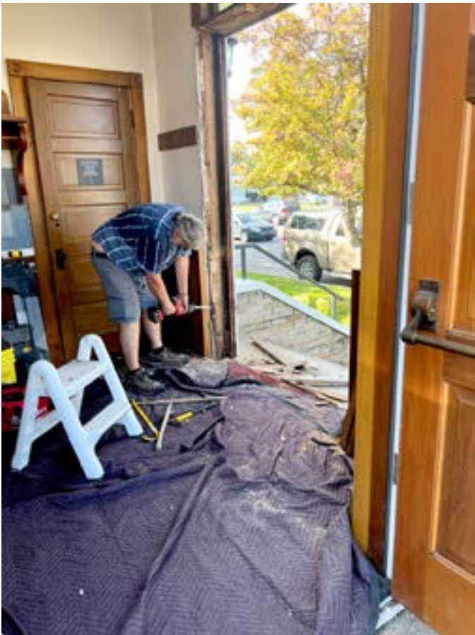
Jerry from Miller, Poineau and Naumes works on preparing the entrance to narthex for our new front doors.
